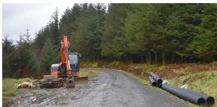
The woody debris dams are constructed (left) to slow the flow of water. Culverts are installed (above) to spread water over land rather than go into the watercourses. The Pennal forestry workers' car park (below, left) has been upgraded for public use.
